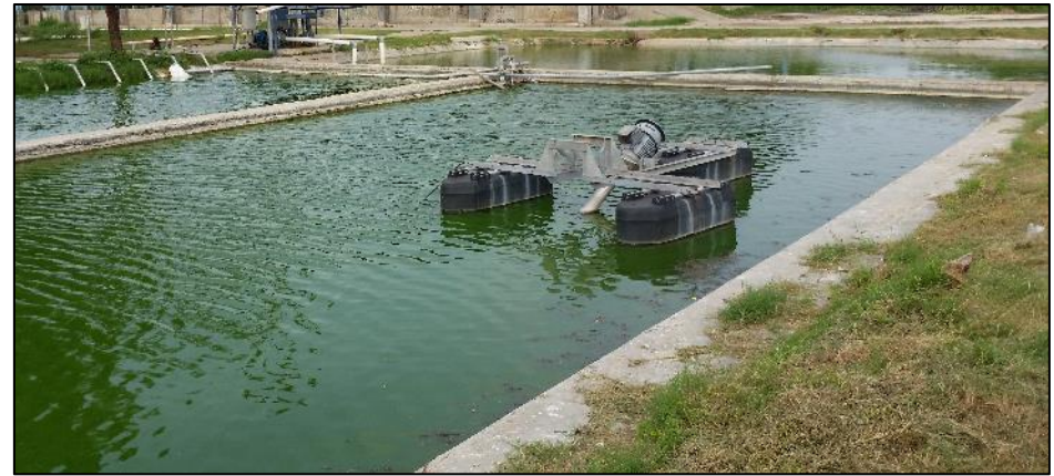
One Aerator for large pond
