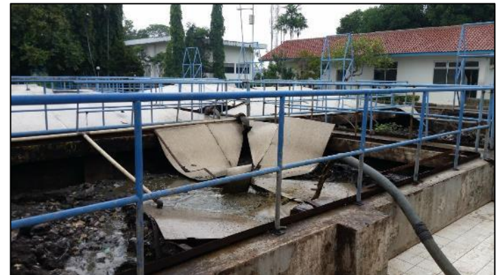
Bypassing initial grit removal due to broken mechanical equip.
