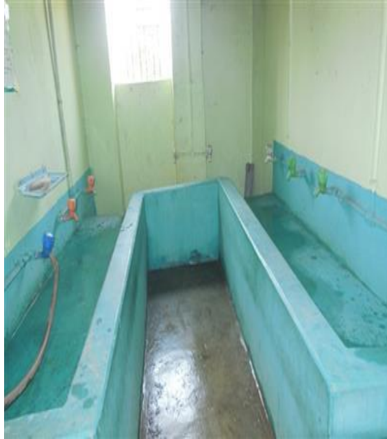
Taps at each handwashing unit
