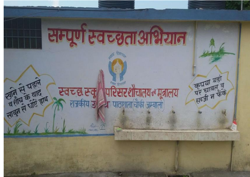
Running water with taps at all handwashing points
